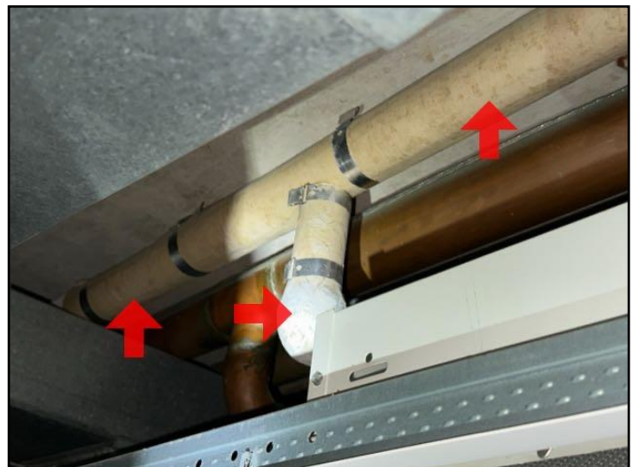
Possible asbestos containing materials
