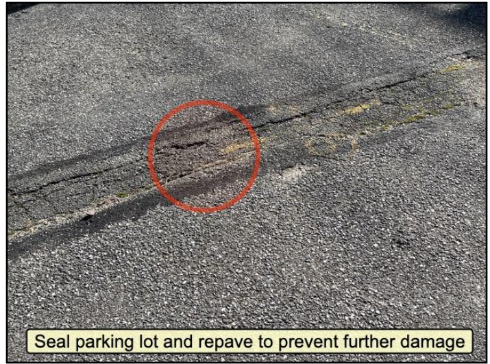
Cracked or damaged surfaces
