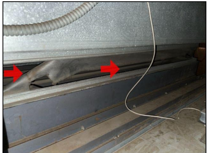
Disconnected or leaking
