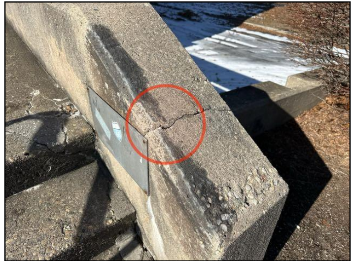
Masonry or concrete cracking
