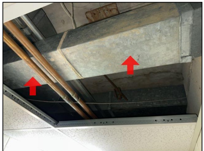
Older uninsulated ducts
