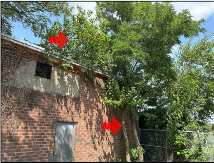
Trees or shrubs too close to building
