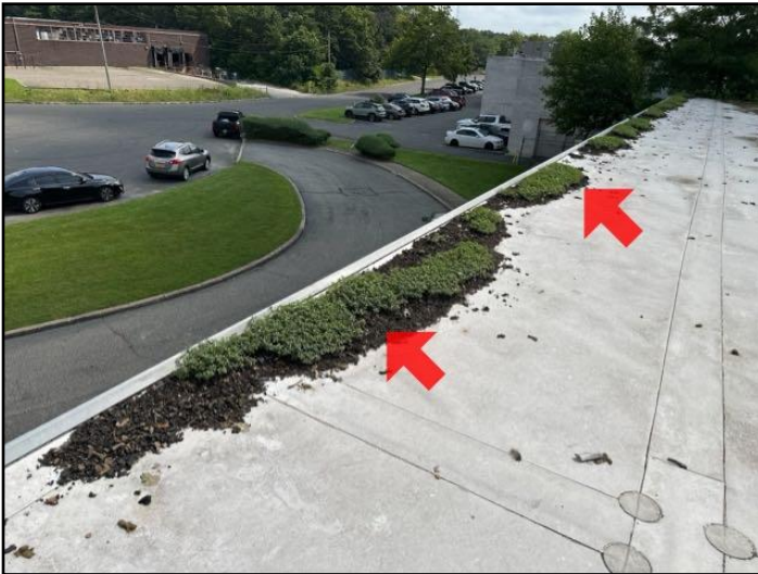
Debris/oil on roof
