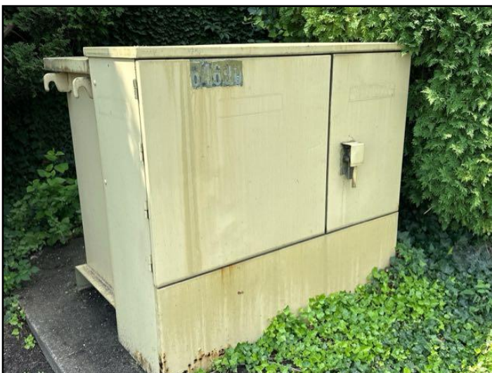
General view of electrical
