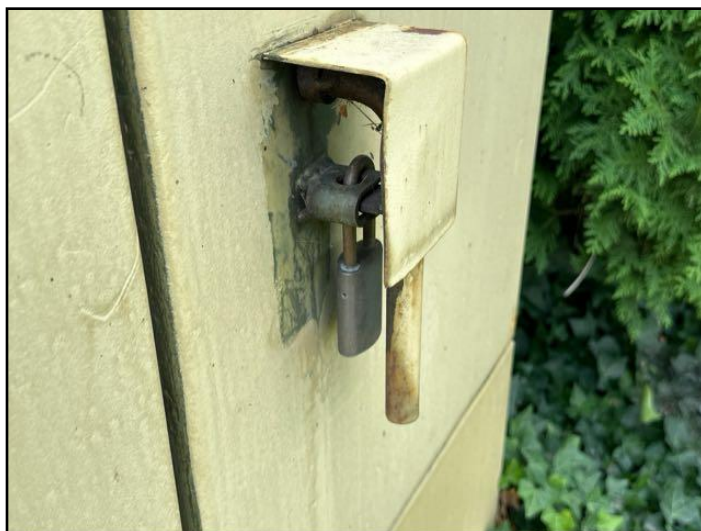
General view of electrical
