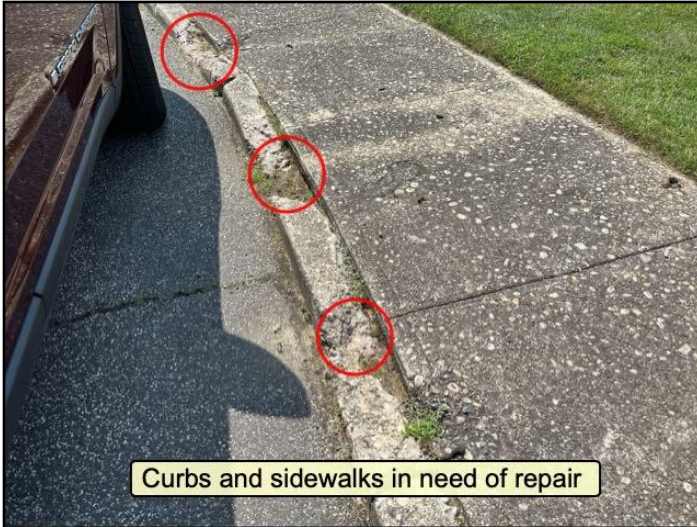
Parking lot cracked/ damaged surfaces
