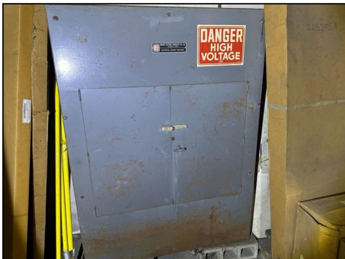
General view of electrical
