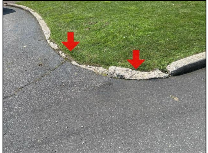
Parking lot cracked/ damaged surfaces
