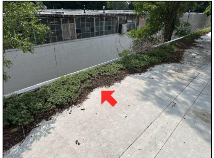
Debris/oil on roof
