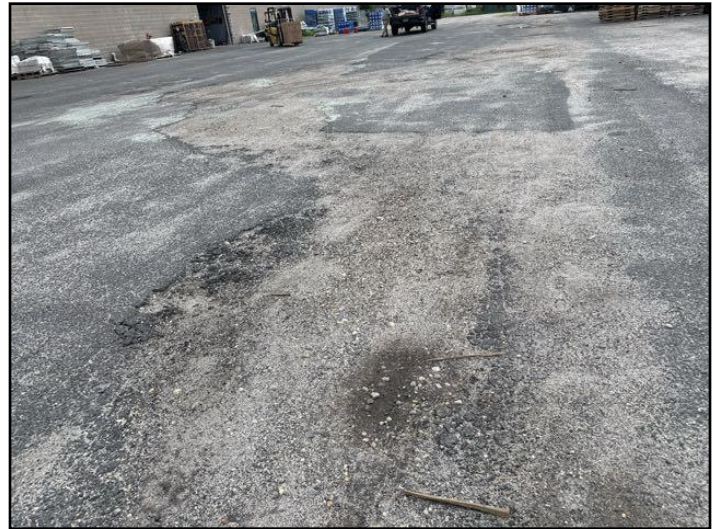
Parking lot surface cracks/ damage
