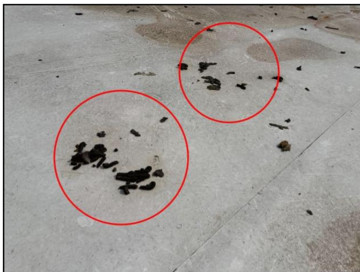
Debris/oil on roof
