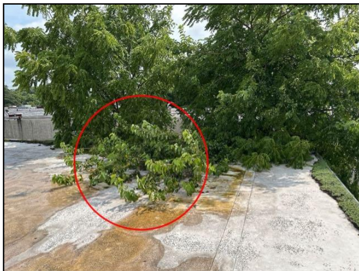
Tree branches touching roof
