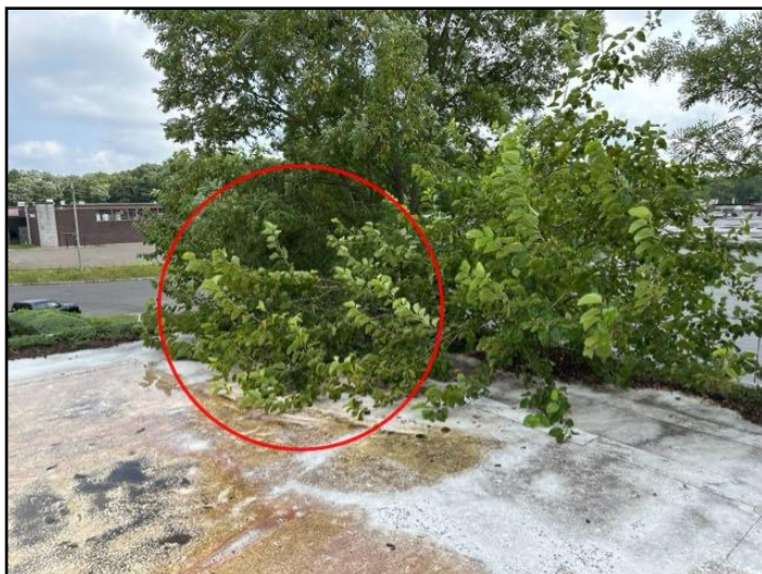
Tree branches touching roof
