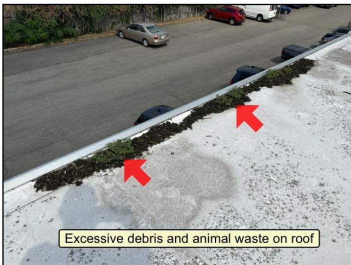
Debris/oil on roof
