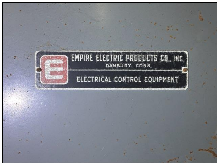
General view of electrical
