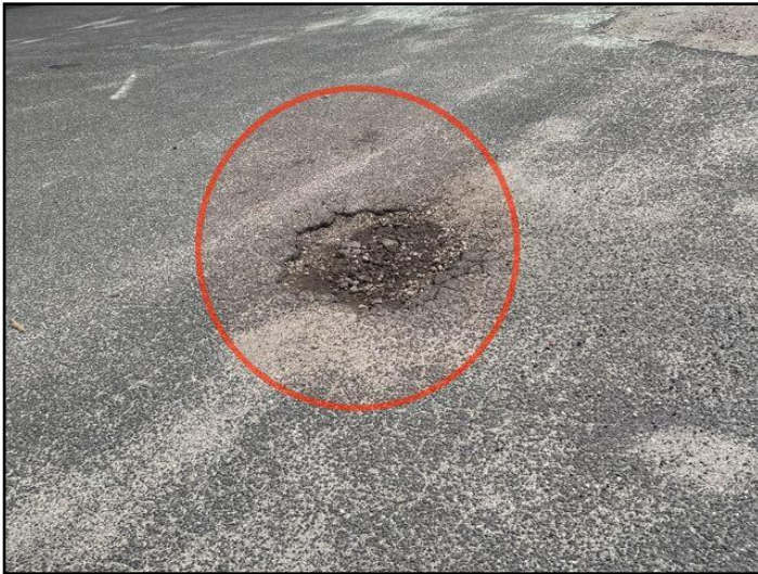
Parking lot surface cracks/ damage
