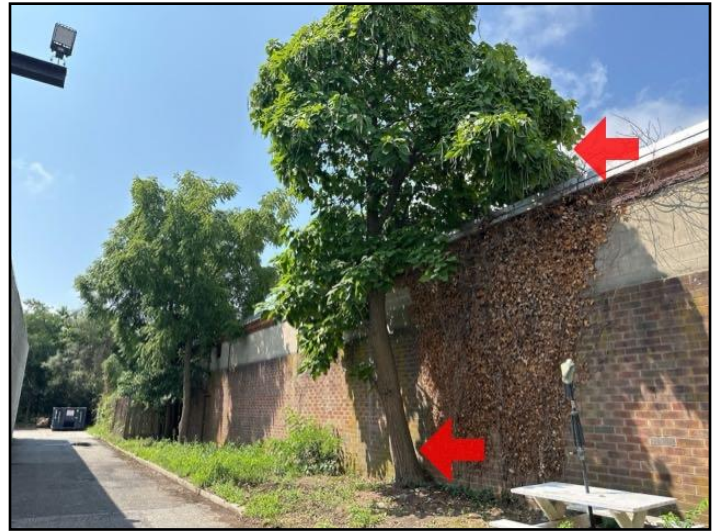
Trees or shrubs too close to building
