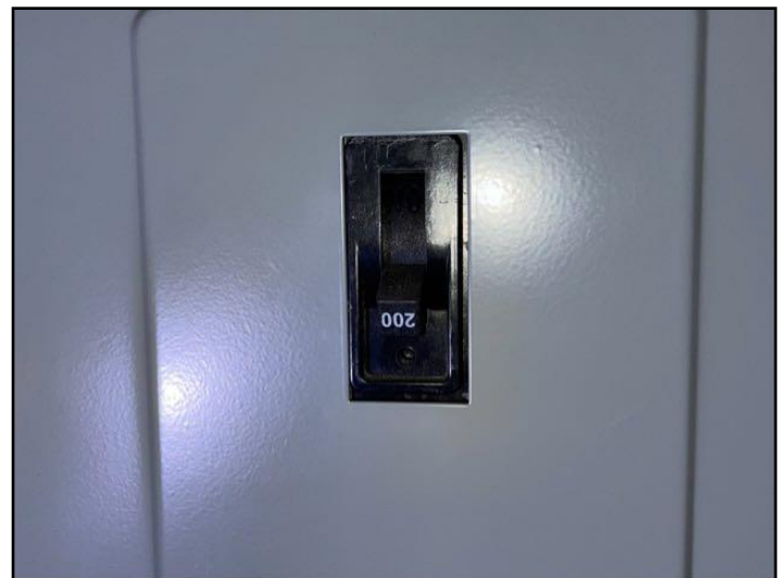
General view of electrical
