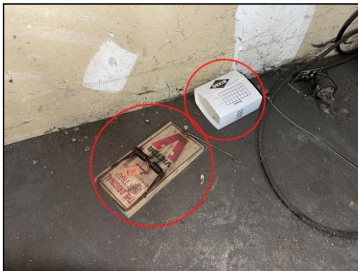
Evidence of rodent activity
