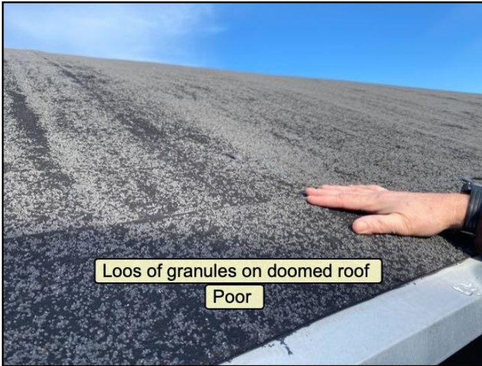
Loss of granules - Poor
