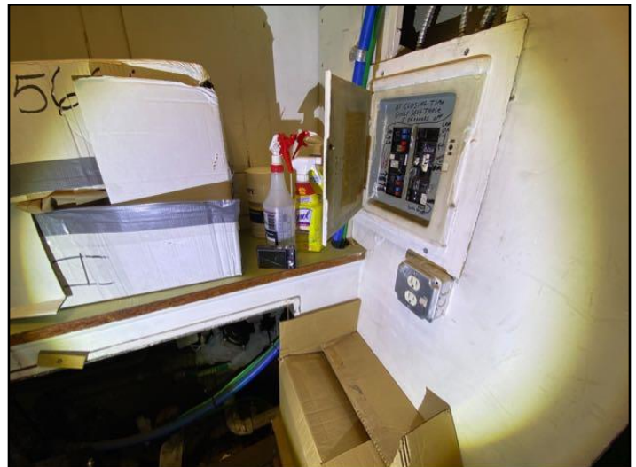
Breakers - utility room
