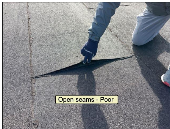
Openings at seams or flashings
