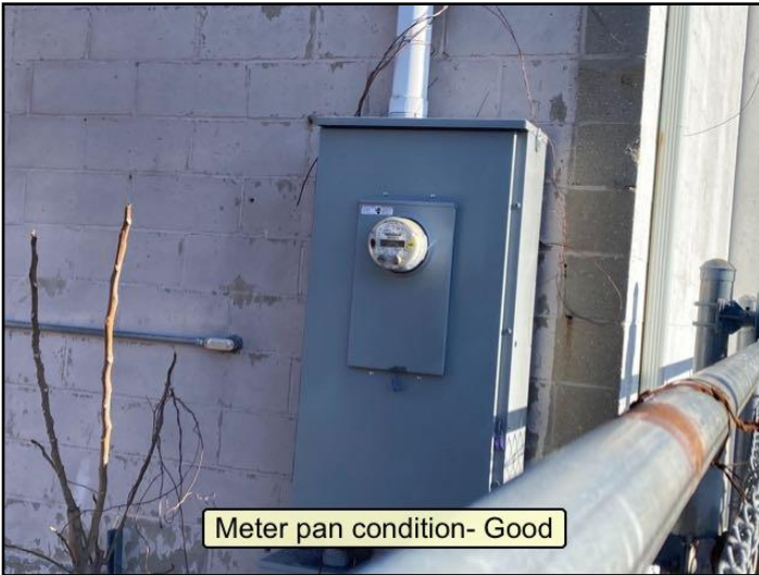
General view of electrical
