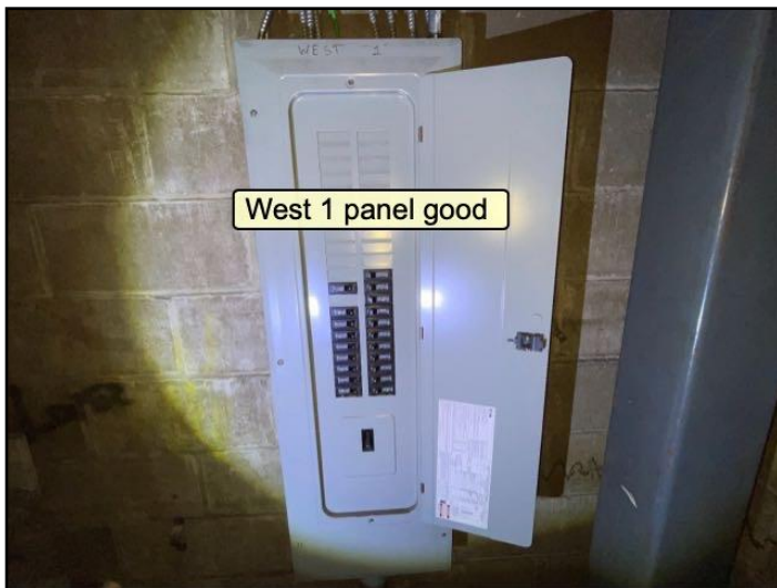
General view of electrical
