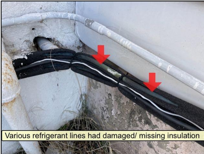
Insulation - missing/ damaged
