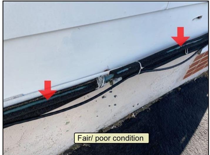
Insulation - missing/ damaged
