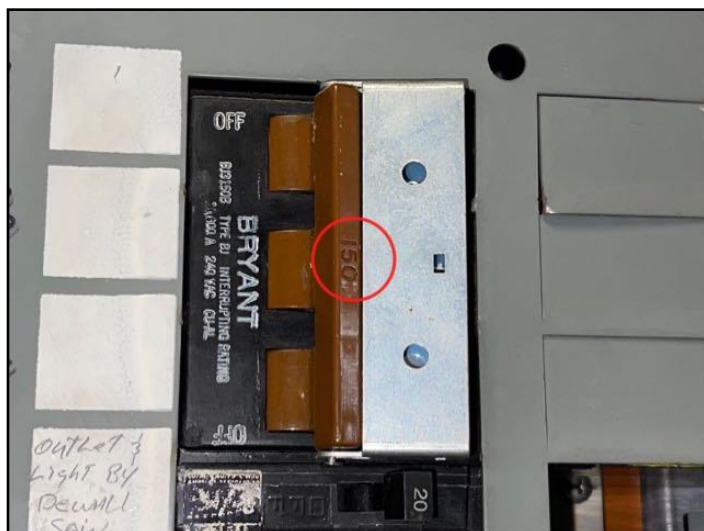
General view of electrical
