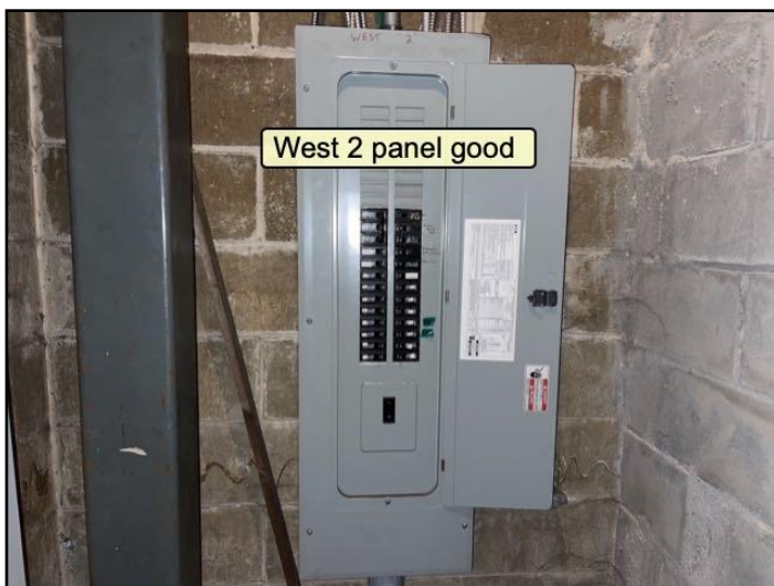
General view of electrical
