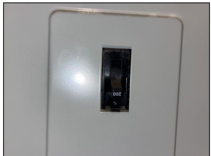
General view of electrical
