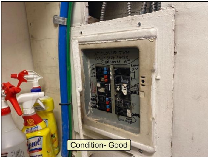
Breakers - utility room
