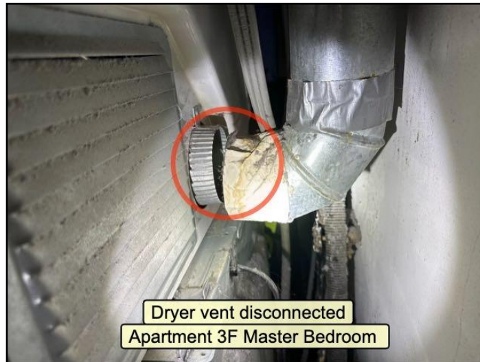
Dryer vent disconnected
