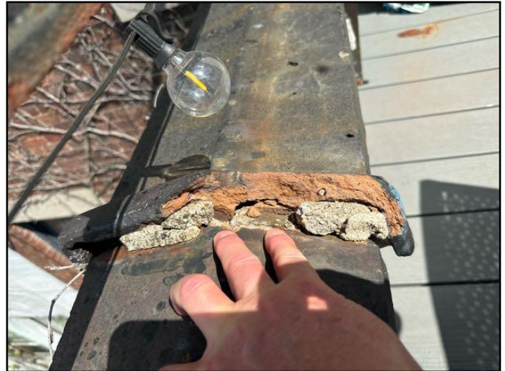
Parapet wall coping damaged
