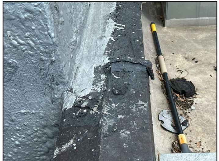
Parapet wall coping damaged
