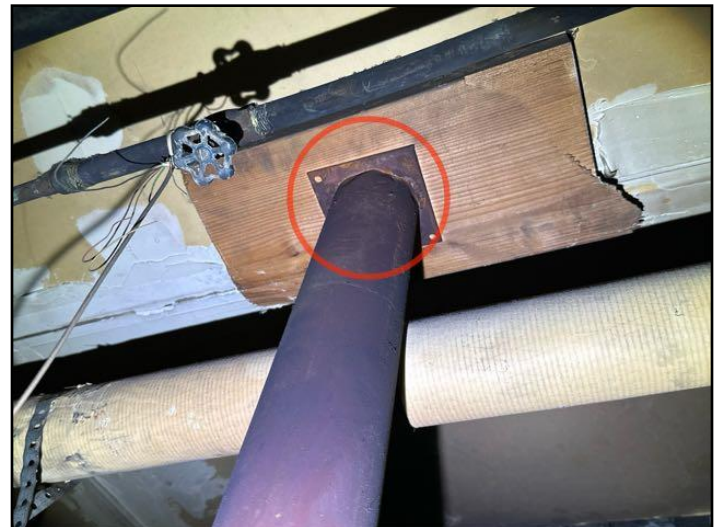
Poorly secured at top or bottom
