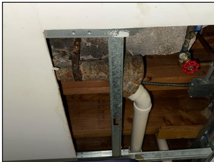
Old galvanized drains
