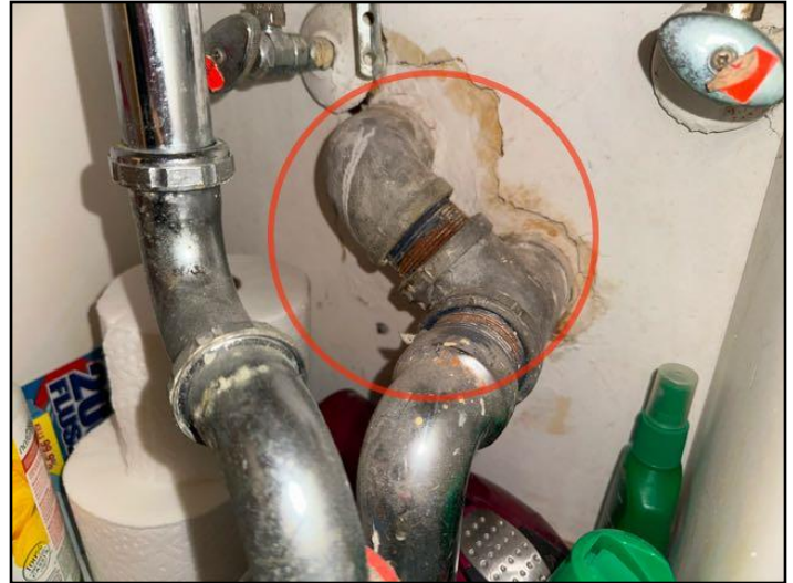
Old galvanized drains
