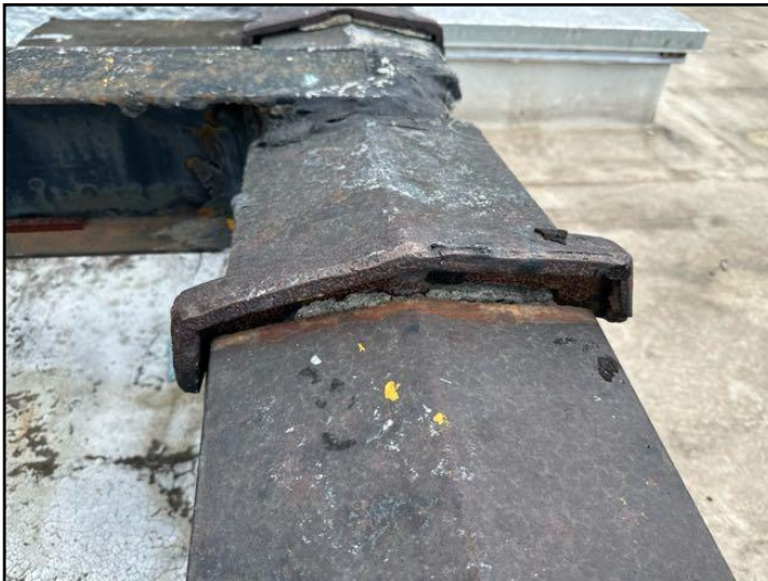
Parapet wall coping damaged
