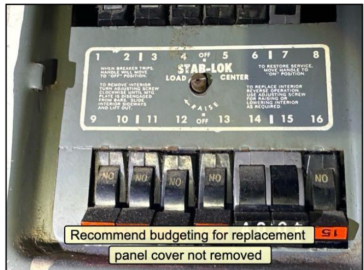
Old Stab-Lock panel and breakers
