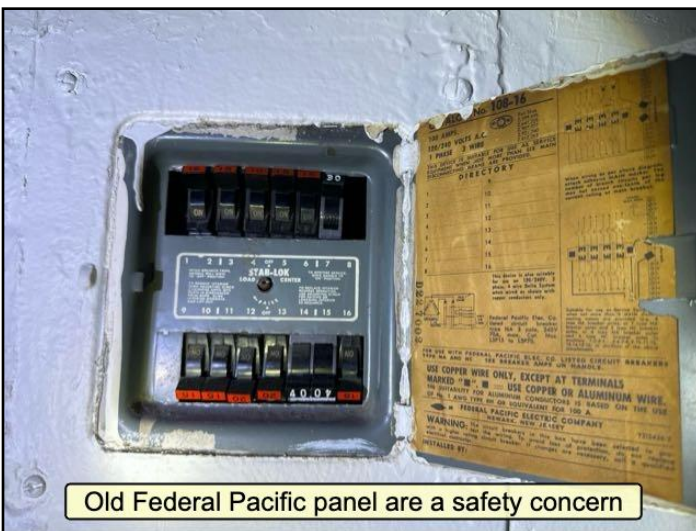
Old Stab-Lock panel and breakers
