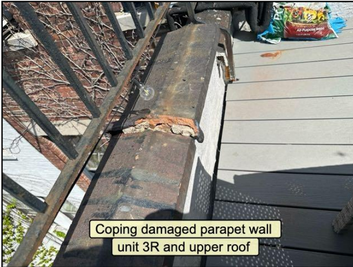
Parapet wall coping damaged
