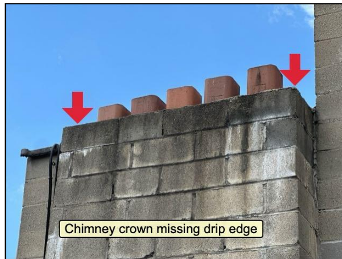
No drip edge on cap (crown)
