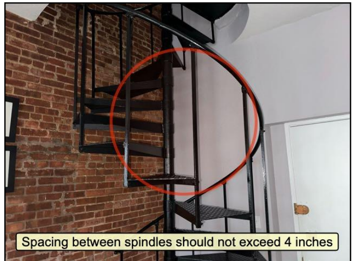
Handrails too wide
