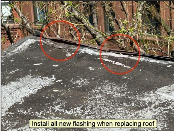
Replace when re-roofing
