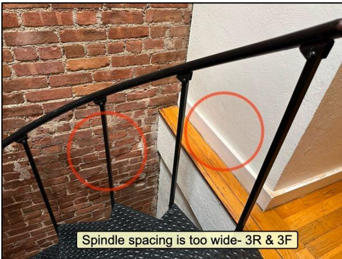
Handrails too wide
