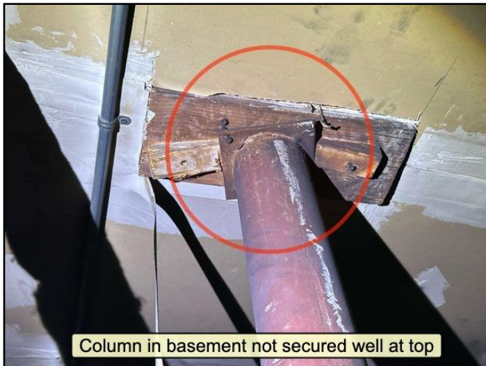
Poorly secured at top or bottom
