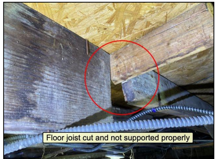
Split or damaged
