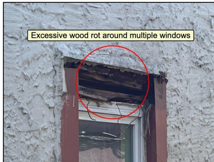
Flashing loose, missing or deteriorated
