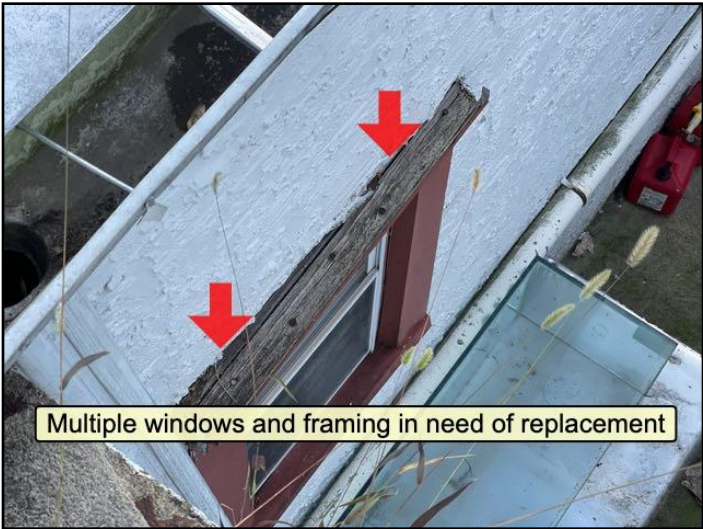
Flashing loose, missing or deteriorated
