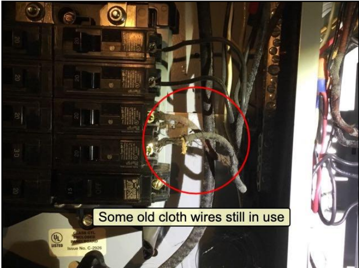
Old cloth wires have tendency to dry out an...
