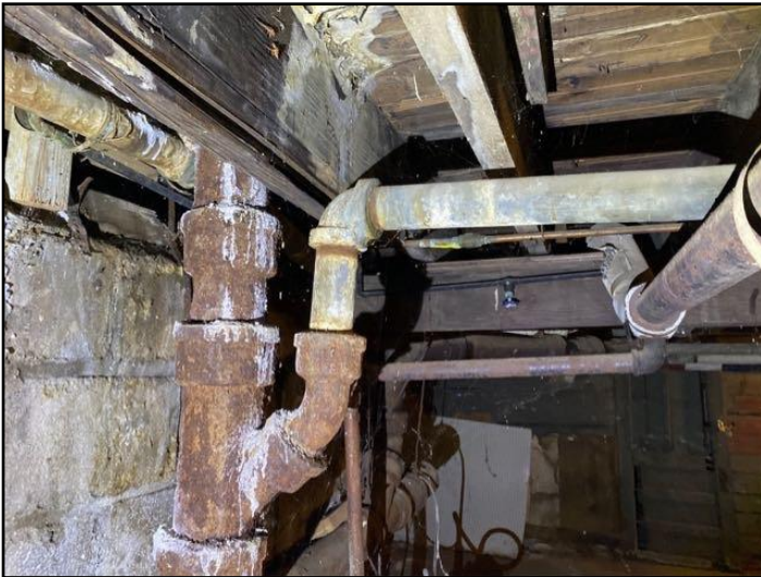
Split, rusted or damaged
