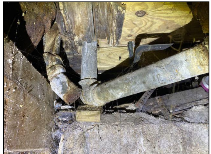
Old galvanized pipes rust from inside out....
