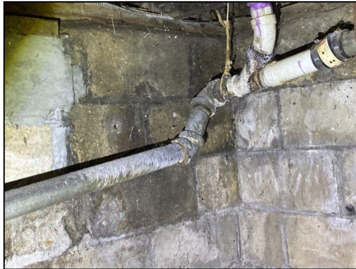
Old galvanized pipes rust from inside out....
