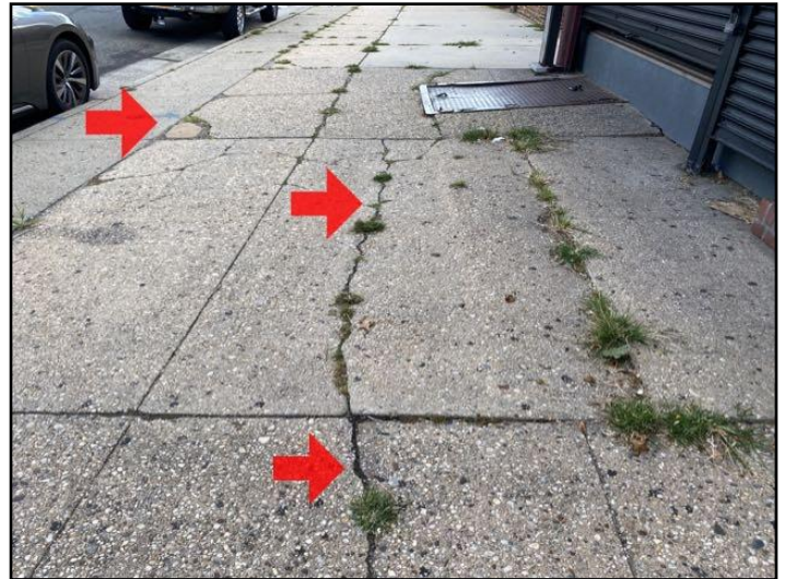
Cracked or damaged surfaces
