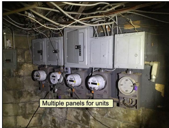
General view of electrical system
