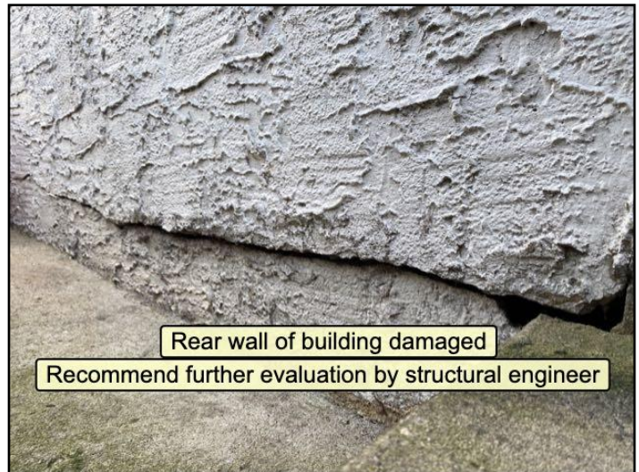
Bowed, bulging or leaning
