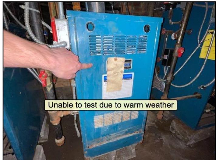
All heating systems need service prior to purchase
