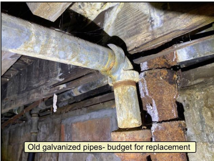
Old galvanized pipes rust from inside out....
