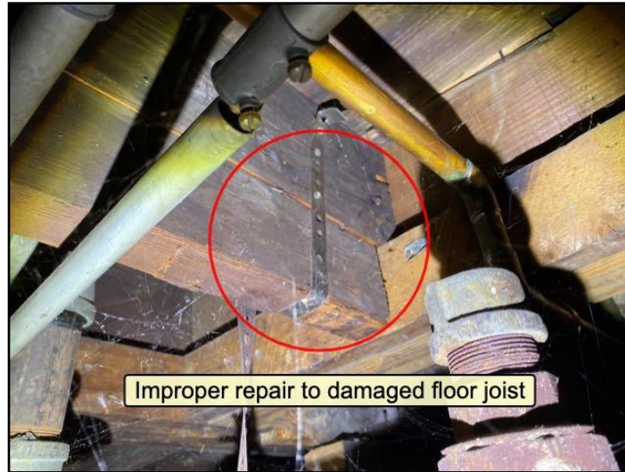
Split or damaged
