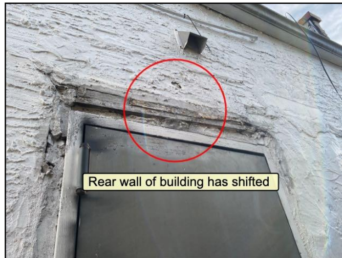
Bowed, bulging or leaning
