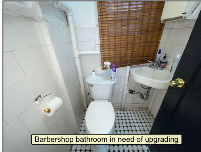
Bathroom in need of upgrading. Recommend...
