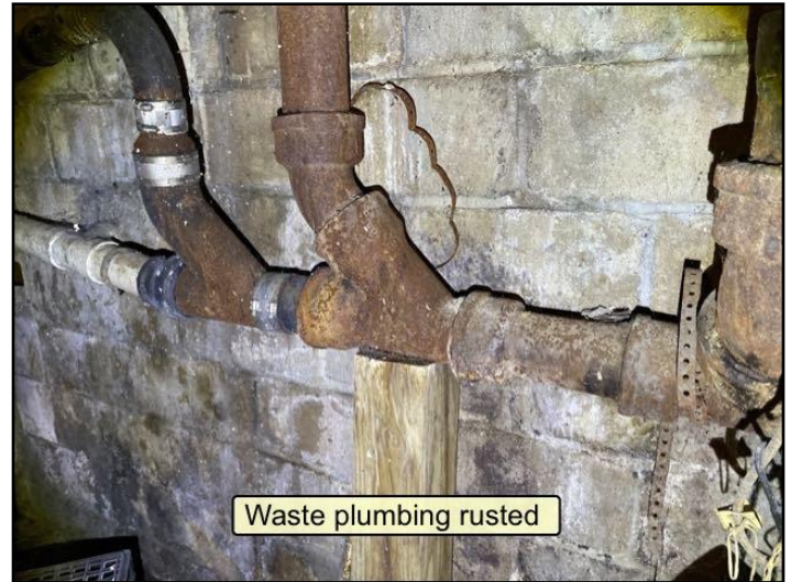
Split, rusted or damaged
