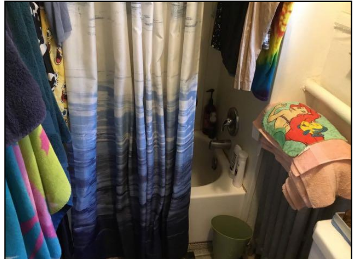
Bathroom in need of upgrading. Recommend...
