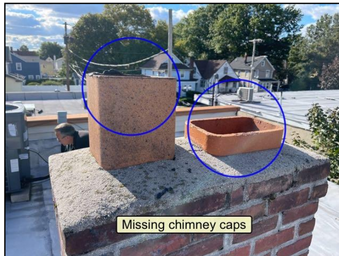
Missing chimney cap
