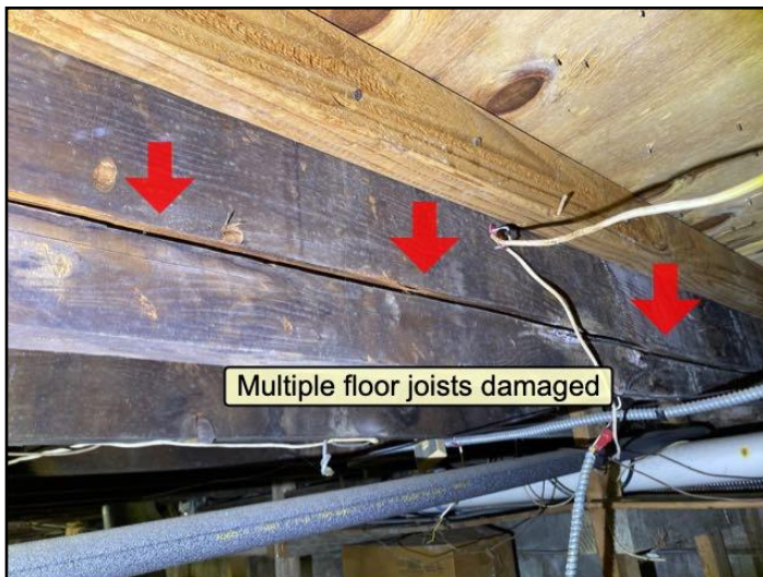
Split or damaged
