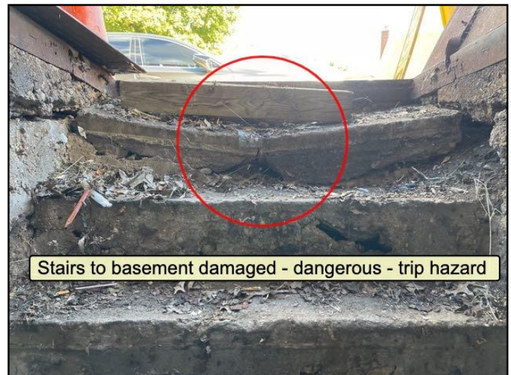
Masonry or concrete cracking
