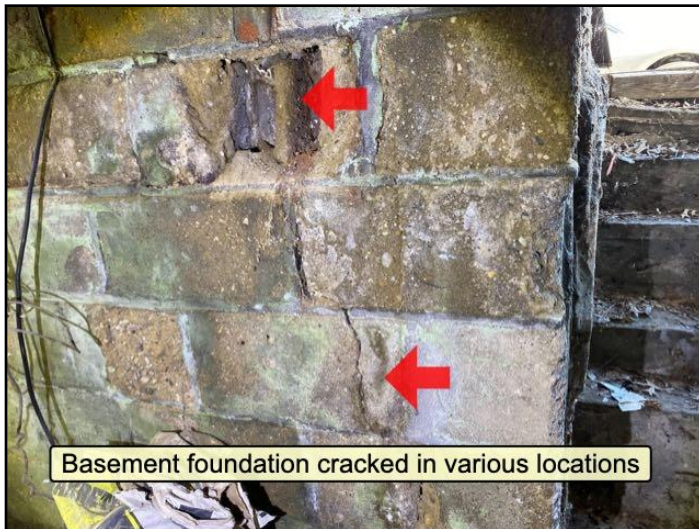
Bowed, bulging or leaning
