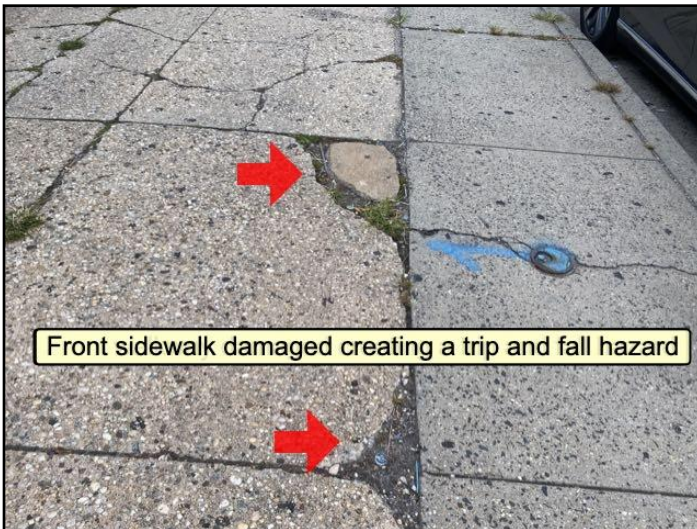
Cracked or damaged surfaces
