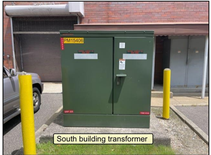
South building transformer
