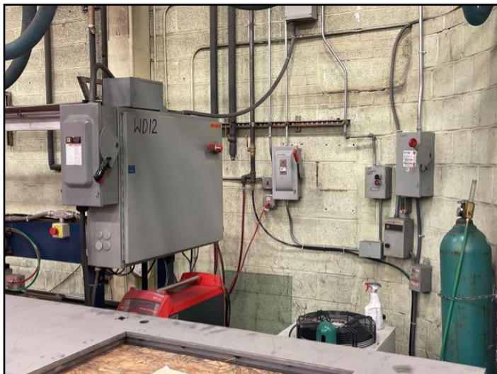
General view of electrical- South Building
