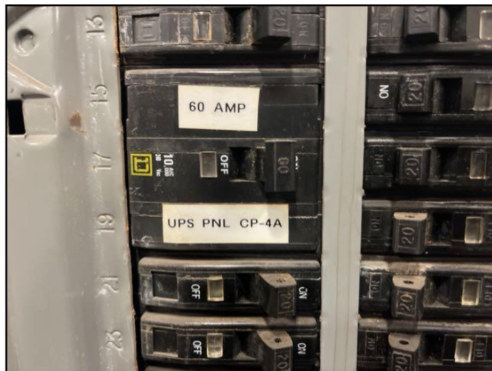
General view of electrical- South Building
