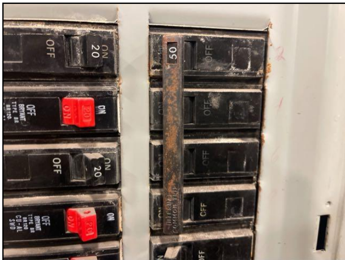
General view of electrical- South Building
