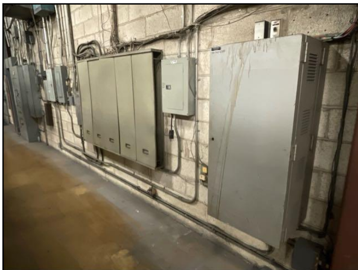
General view of electrical- South Building
