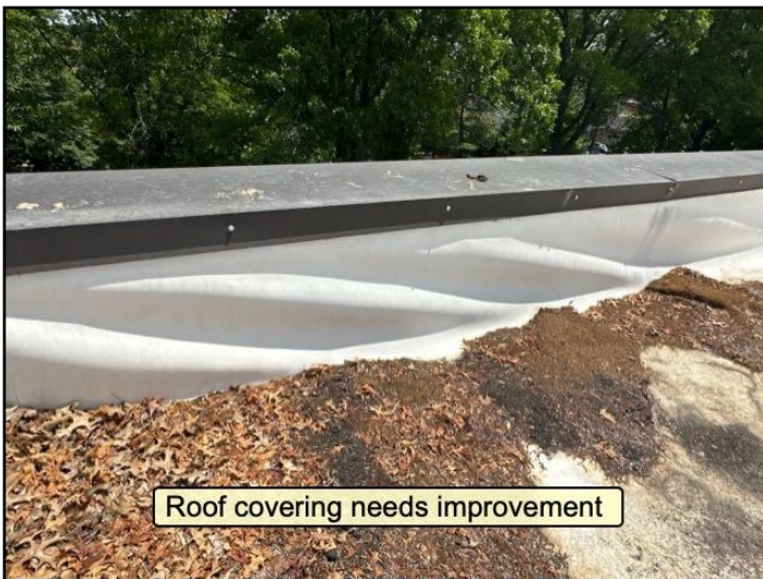
Buckling or wrinkling
