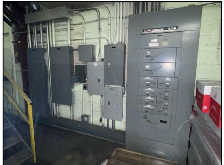
General view of electrical- South Building
