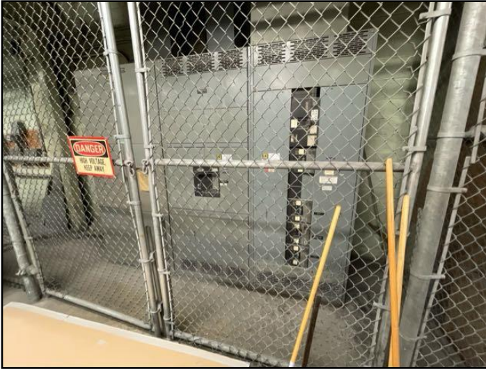
General view of electrical- North Building
