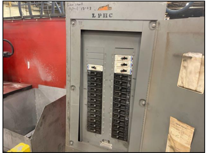
General view of electrical- South Building
