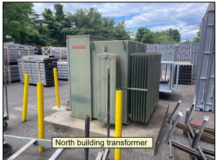
North building transformer
