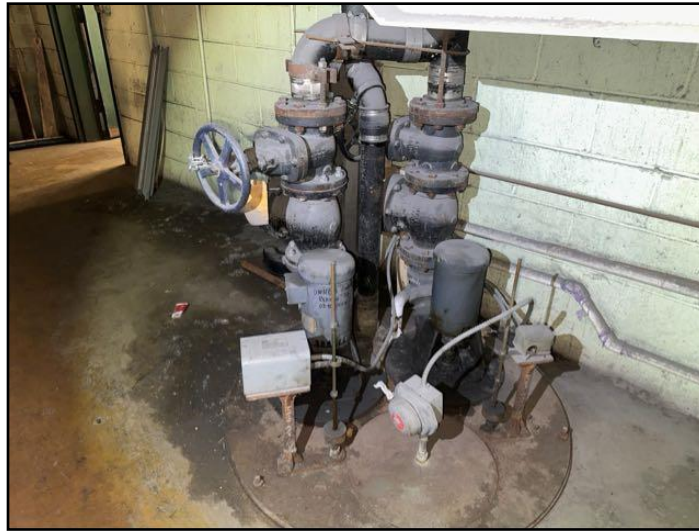
Solid waste pump (ejector pump)
