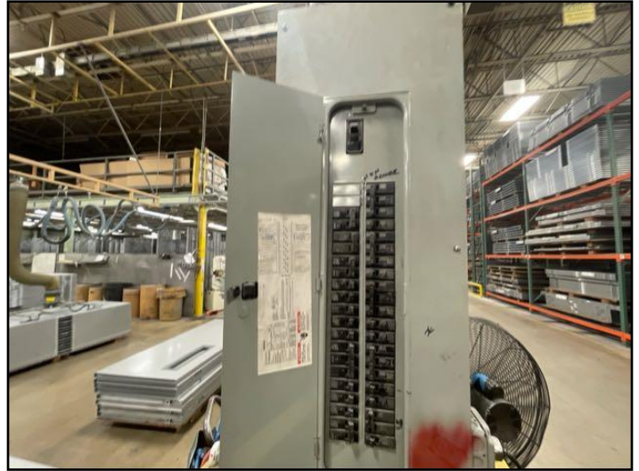
General view of electrical- North Building
