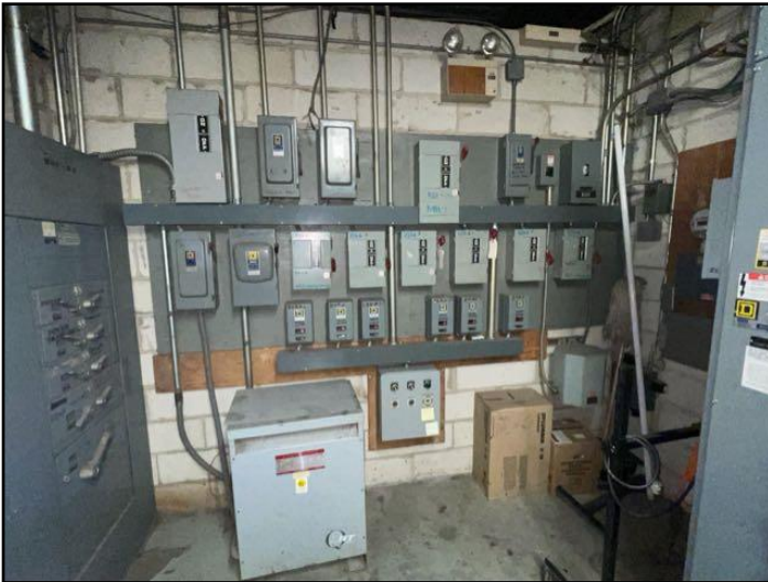
General view of electrical- South Building
