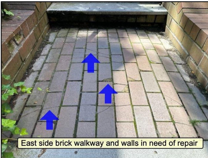
Masonry or concrete cracking
