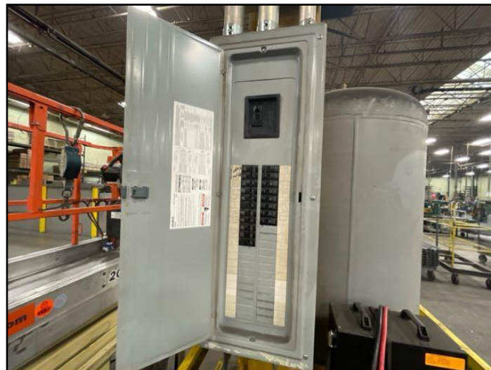
General view of electrical- South Building
