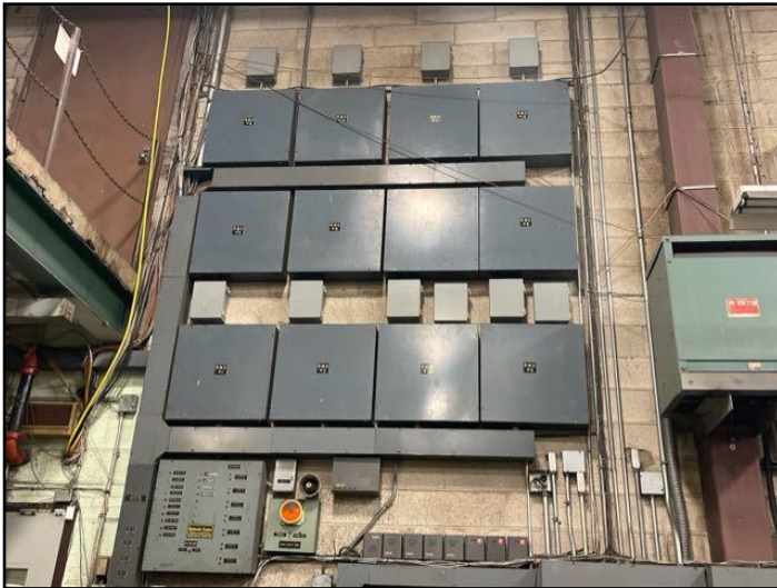
General view of electrical- South Building
