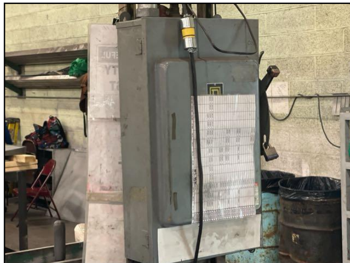
General view of electrical- South Building
