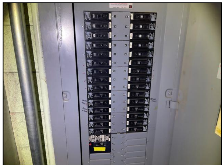
General view of electrical- South Building
