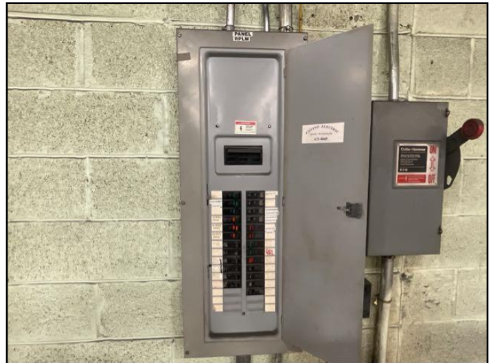
General view of electrical- South Building
