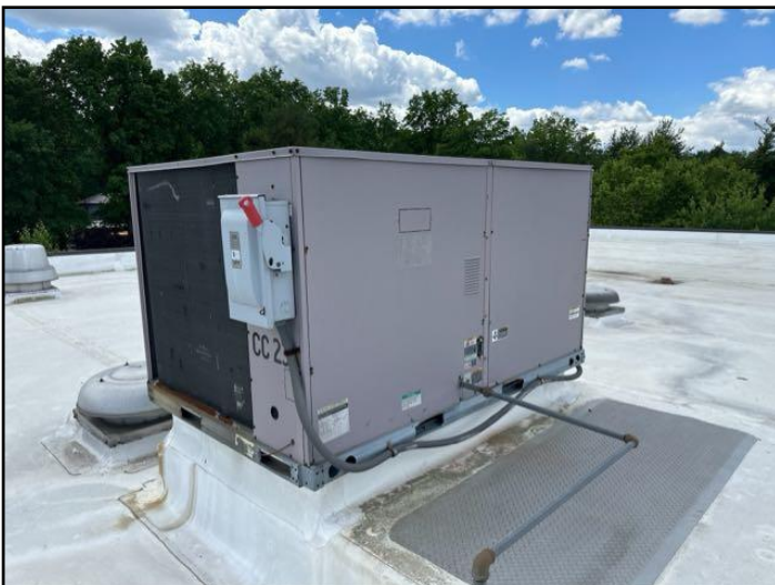
Carrier- Packaged Rooftop Unit (RTU)
