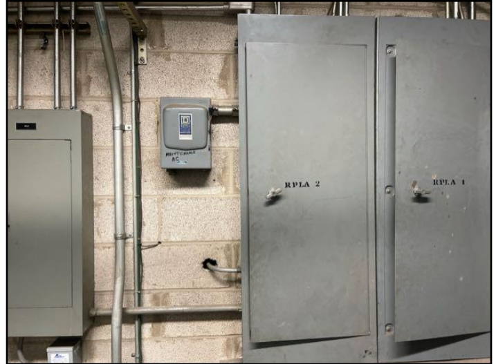
General view of electrical- South Building
