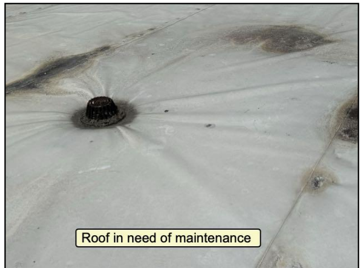
Buckling or wrinkling
