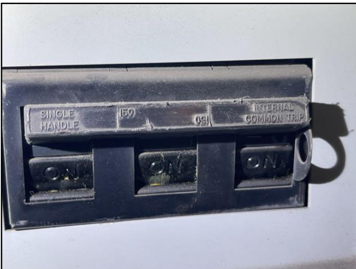
General view of electrical- South Building
