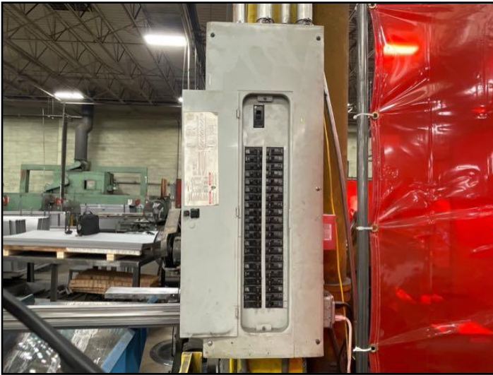
General view of electrical- South Building
