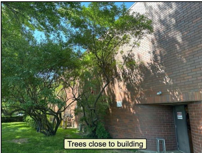
Trees or shrubs too close to building
