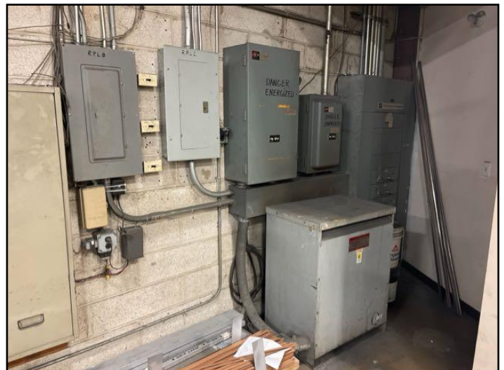
General view of electrical- South Building
