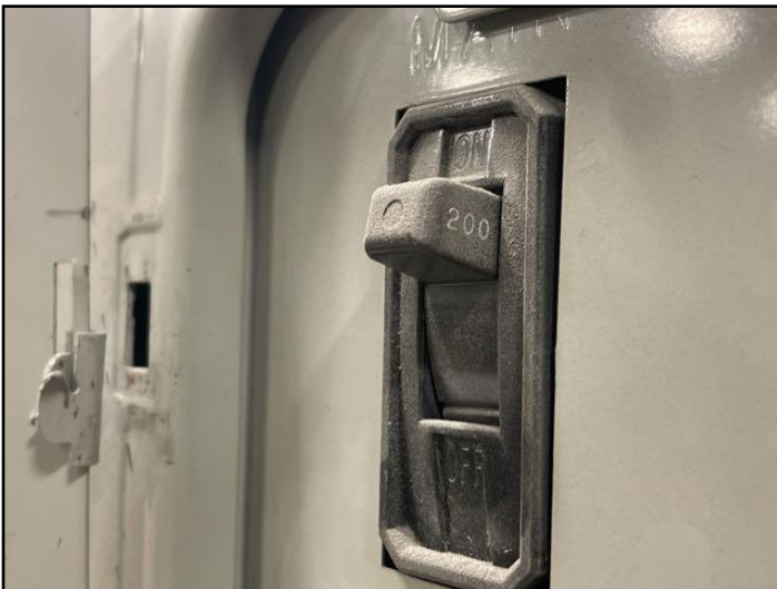
General view of electrical- North Building
