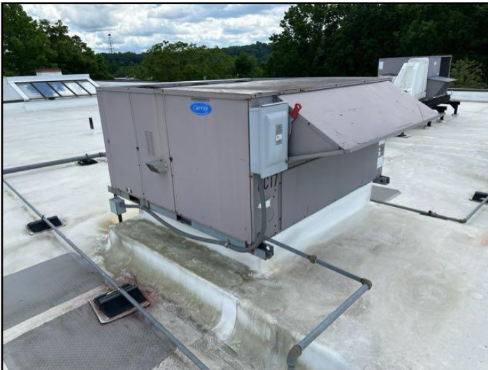
Carrier- Packaged Rooftop Unit (RTU)
