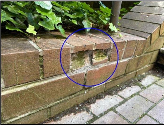
Masonry or concrete cracking
