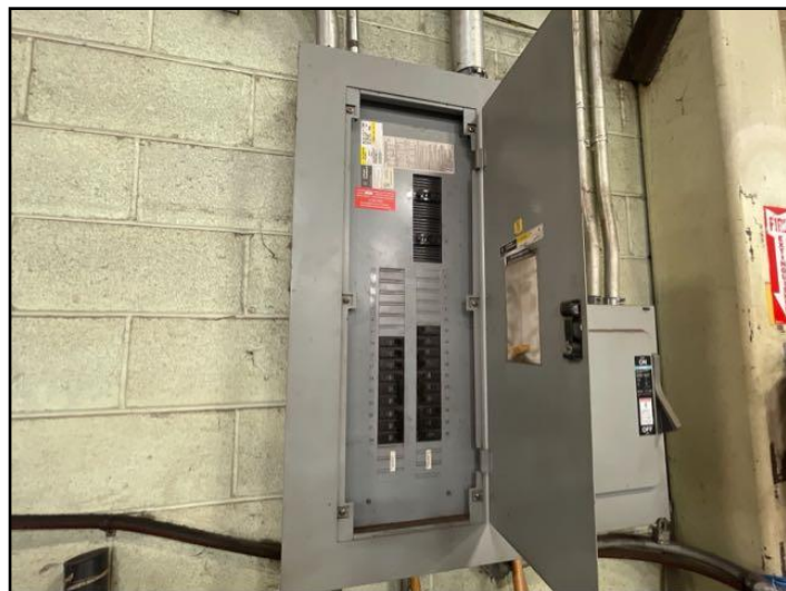
General view of electrical- North Building
