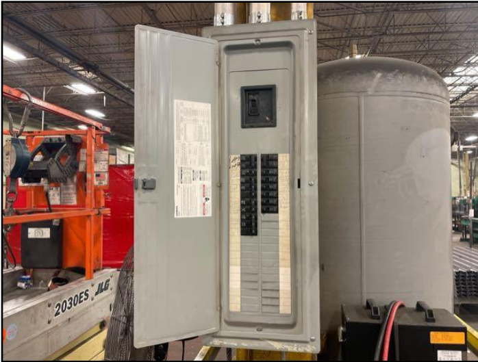
General view of electrical- South Building
