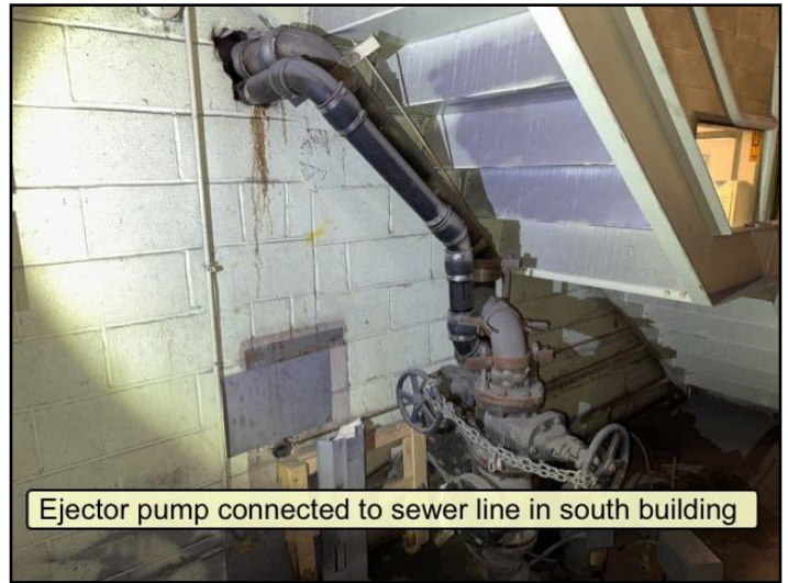
Solid waste pump (ejector pump)
