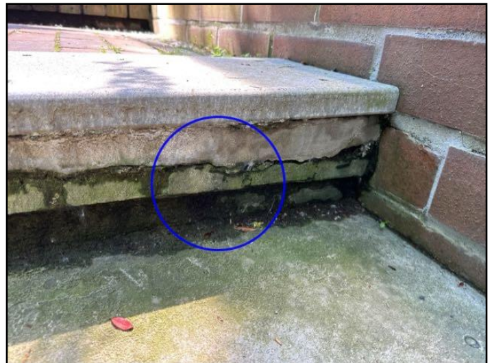
Masonry or concrete cracking
