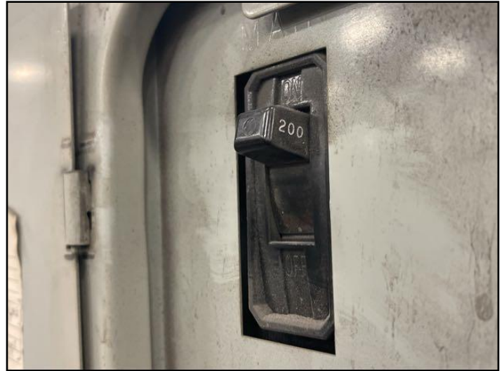
General view of electrical- South Building
