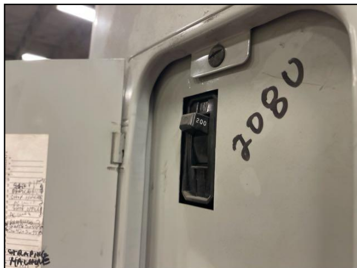
General view of electrical- South Building
