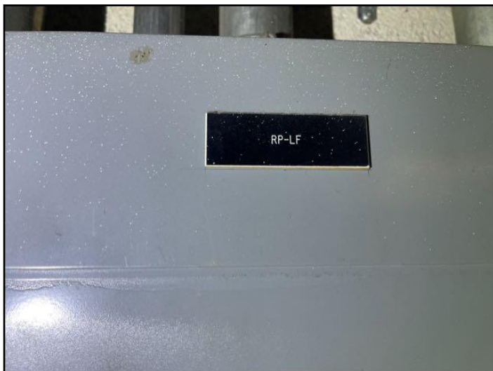
General view of electrical- South Building
