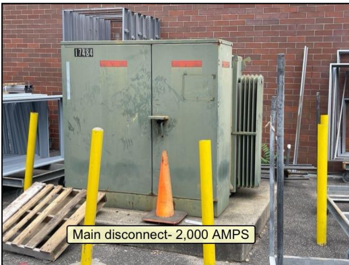
Main disconnect- 2,000 AMPS
