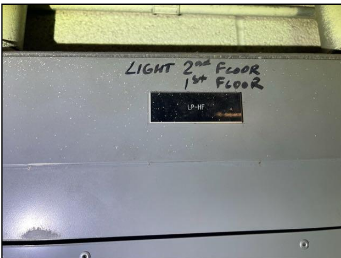
General view of electrical- South Building
