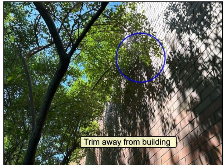
Trees or shrubs too close to building
