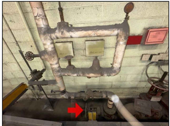
Interior main shut off valve located in south warehouse
