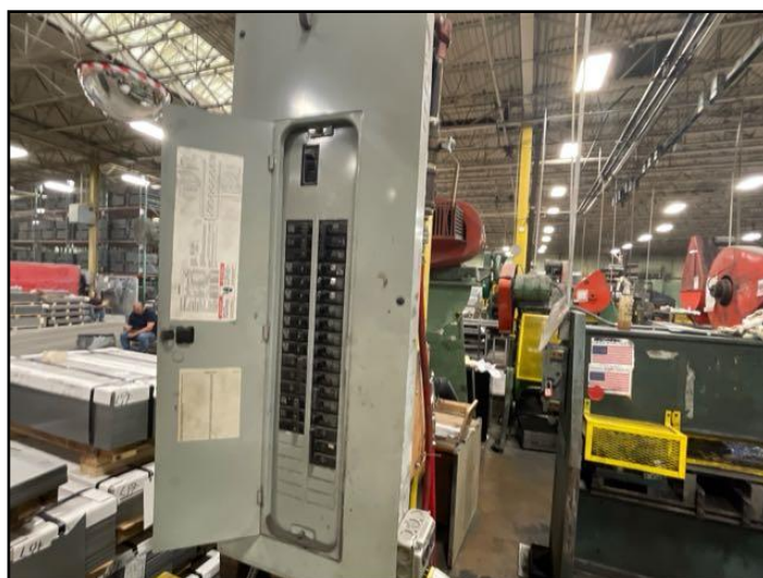
General view of electrical- North Building
