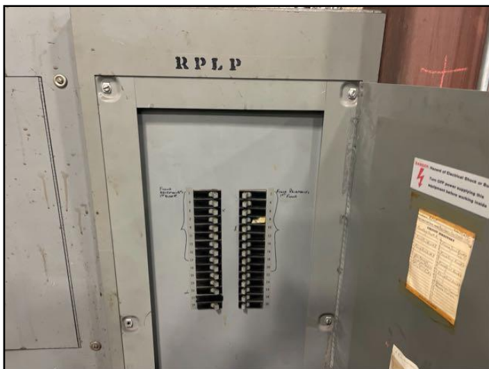
General view of electrical- South Building
