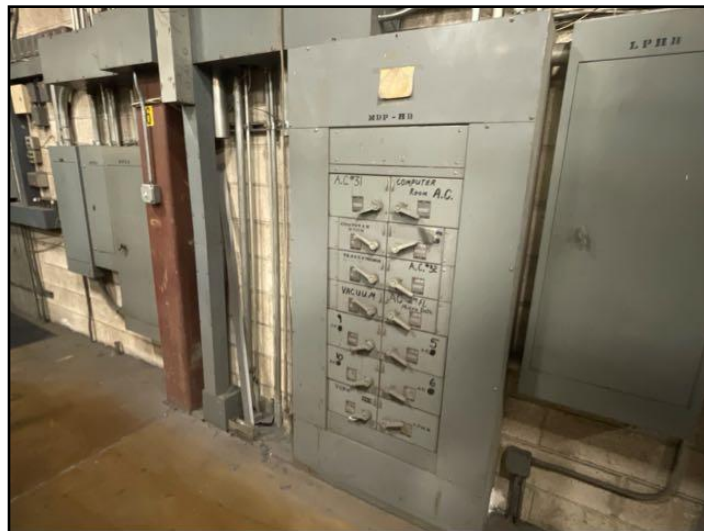
General view of electrical- South Building
