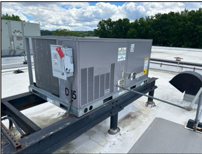
Carrier- Packaged Rooftop Unit (RTU)
