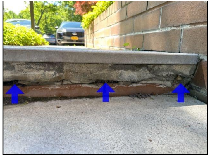
Masonry or concrete cracking
