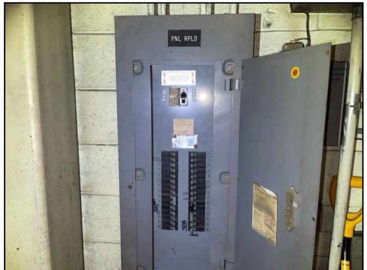
General view of electrical- North Building
