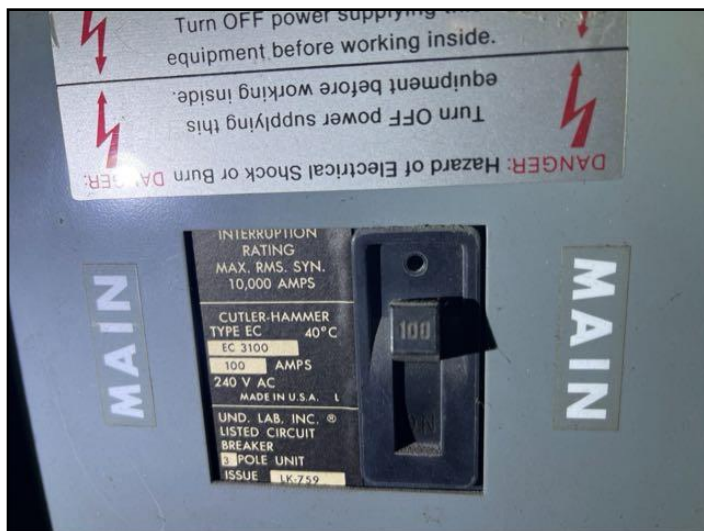
General view of electrical- North Building
