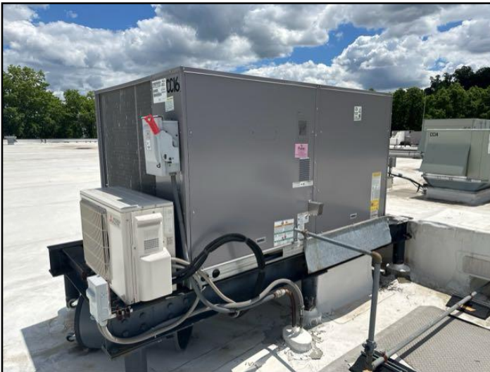
Carrier- Packaged Rooftop Unit (RTU)
