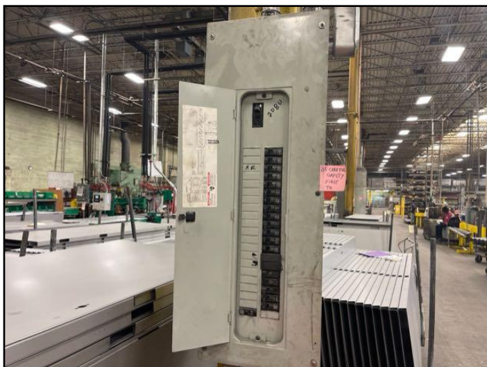
General view of electrical- South Building
