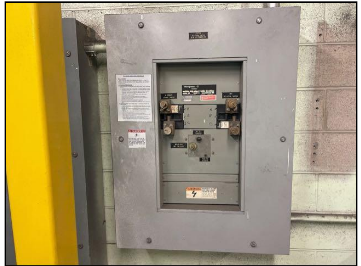
General view of electrical- South Building
