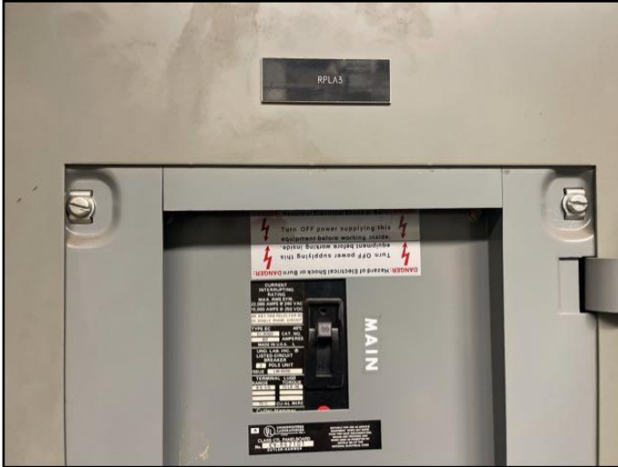
General view of electrical- South Building
