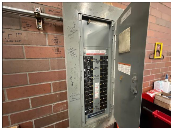
General view of electrical- North Building
