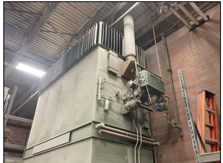
General view of heating
