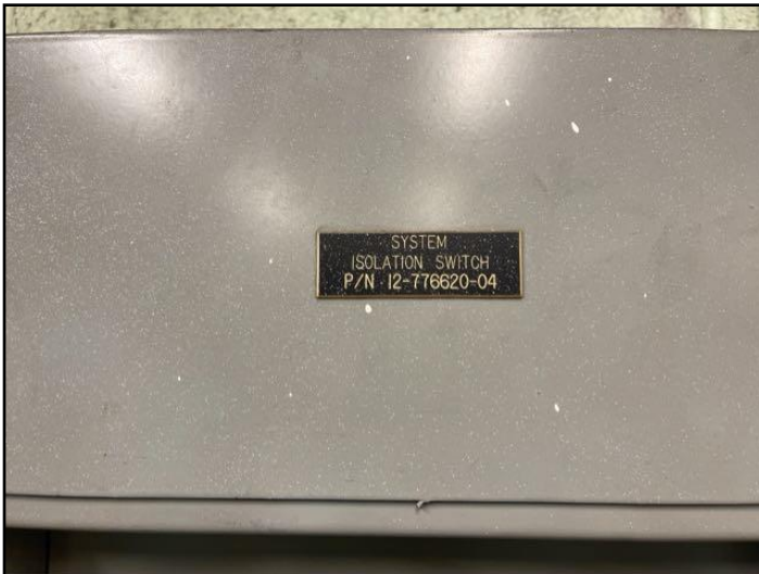
General view of electrical- South Building
