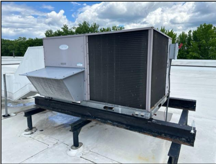
Carrier- Packaged Rooftop Unit (RTU)
