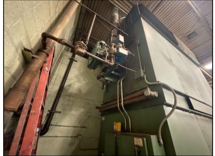
General view of heating
